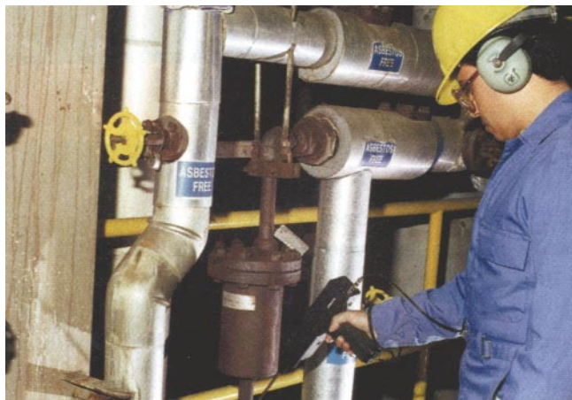
Fig. 1. In the hands of experienced technicians, ultrasound equipment can provide accurate analysis of steam trap operations.
