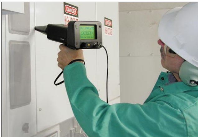
Figure 2. Handheld ultrasonic monitors are used to detect ultrasonic emissions produced by arcing, tracking, and coronas in an electric cabinet. The operator first checks door seams and air vents for airborne signals. If there are no air paths, the sensor's waveguide is used to probe around the cabinet wall. For continuous monitoring, an ultrasonic unit can be mounted inside the cabinet.
