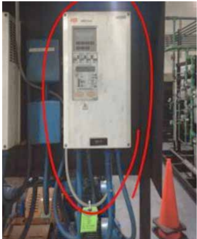
Picture of Leak
