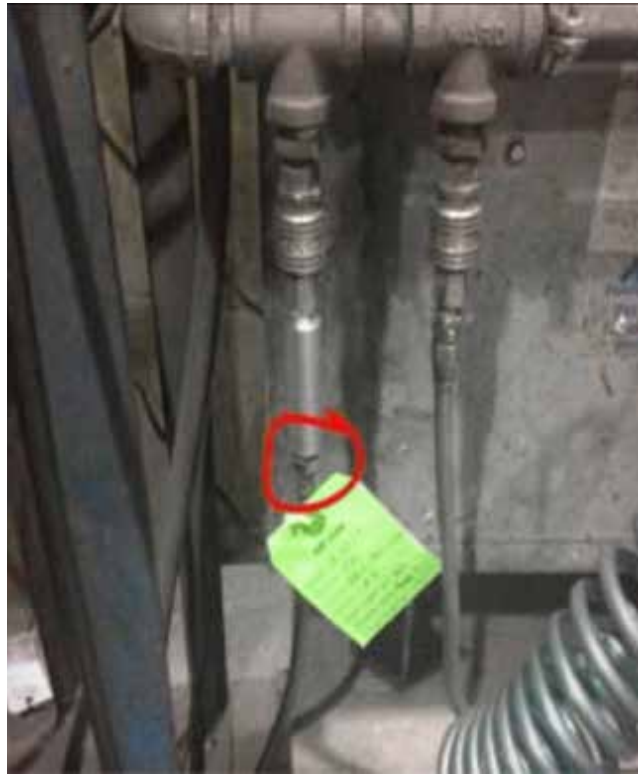
Picture of Leak
