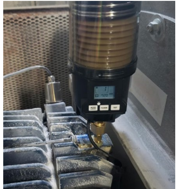
Figure 1 OnTrak SmartLube system installed monitoring the real-time lubrication needs and health of the bearing on an air handler motor.
