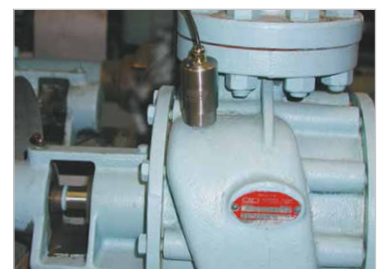
Monitor cavitation, bearings, and valves
