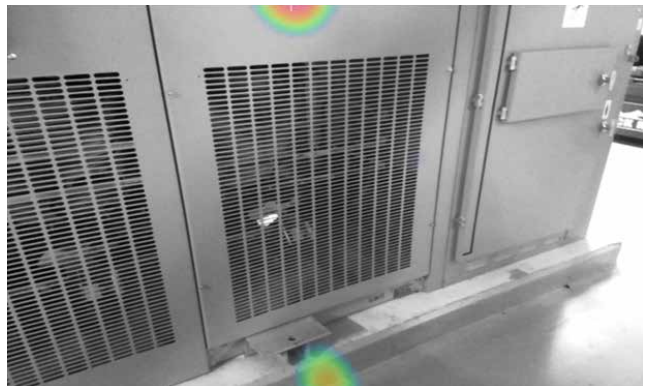
The UltraView Camera (Si124) report after the fix. There is no partial discharge located on the transformer.
