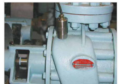
Monitor cavitation, bearings, and valves
