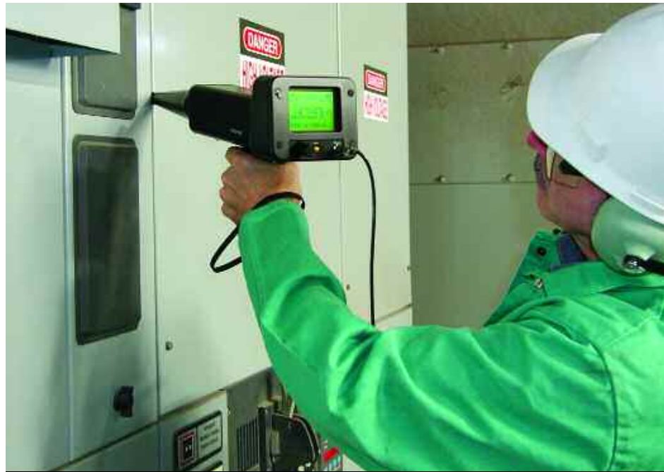
Excessive heat indicates component failure, especially the degradation of electrical contacts that may be hidden behind enclosures.
