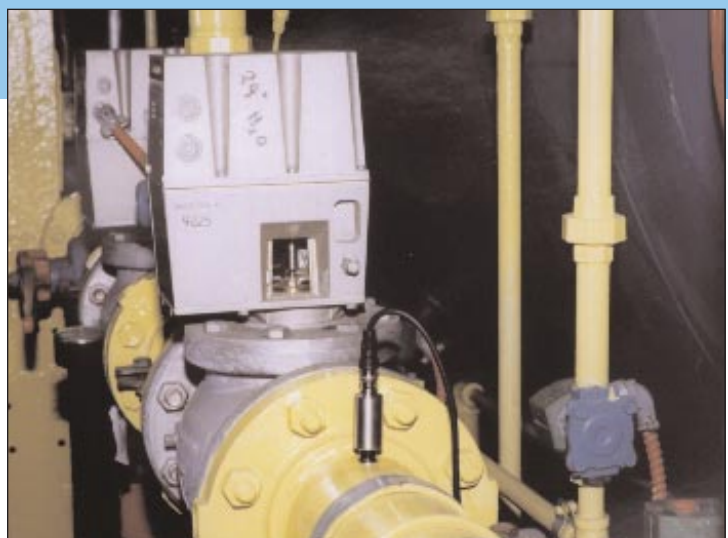
Valve flow / no flow condition monitoring.
